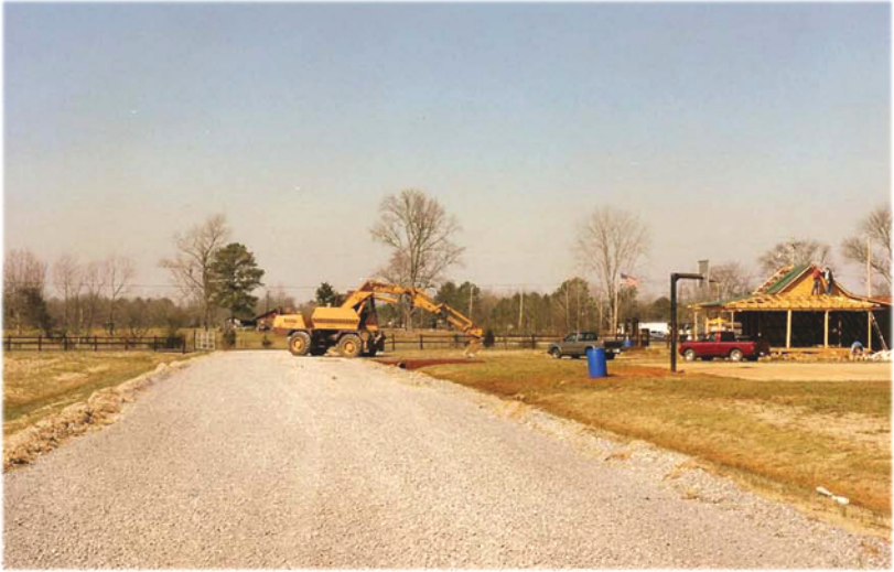
Working on Visitor's Center and culvert into entrance. Barrett Shelton, Decatur Daily gave $27,000 to restore the house.
