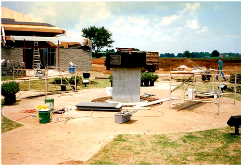
Statue base made of solid concrete with a granite veneer cover and plaque.
