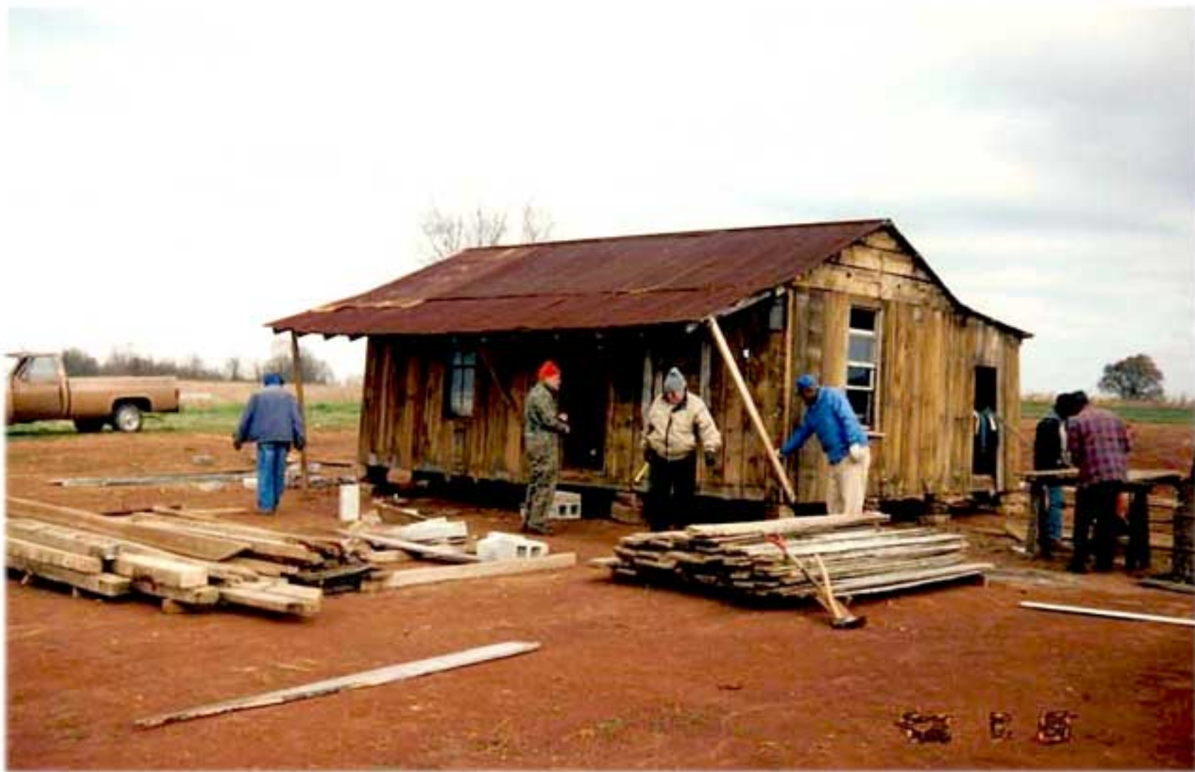
Beginning the work to restore the Home Replica. Left to Right: Buck Reed, Billy Warren Shelton, Curtis Cole and Thurman White
